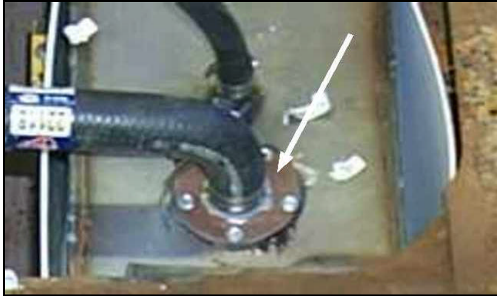
Figure 9: Check valve bolted to the tank.
