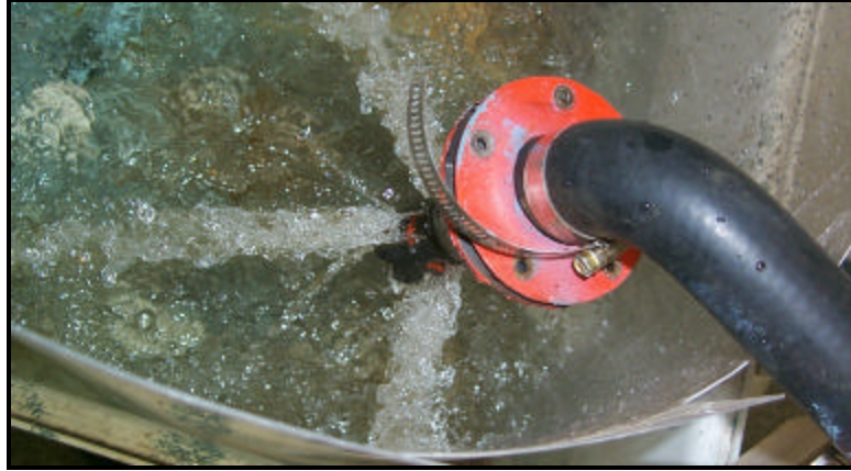
Figure 68: Water draining through the check valve.
