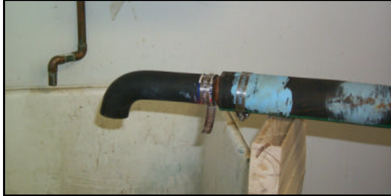
Figure 70: Close-up of the reducer/elbow without the check valve.
