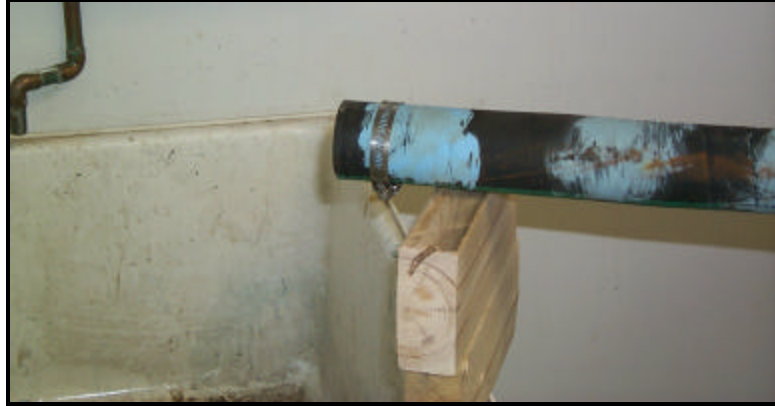
Figure 72: Close-up of the fuel supply tube without reducer elbow or check valve.
